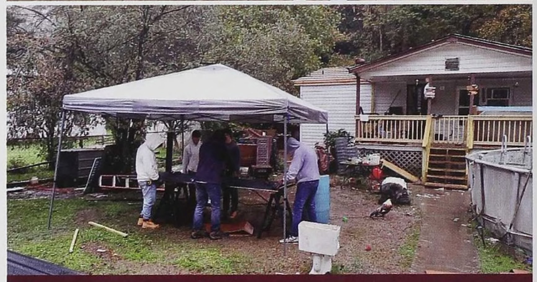
CBA students helped in the construction of a new roof for a house
